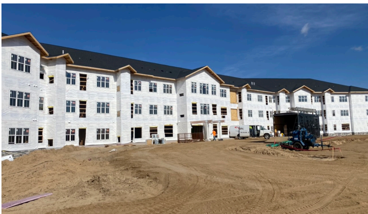
Windows are almost fully in place and soon doors will be on their way to fully enclose the building before winter snow falls (and stays)!
